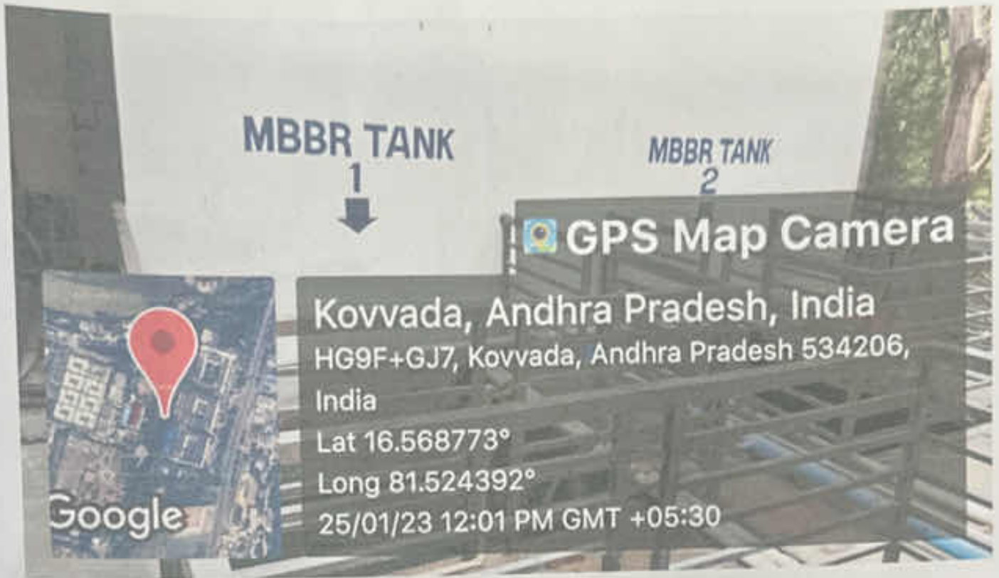
Picture of the domestically used water collecting MBBR tanks in B.V.Raju College
